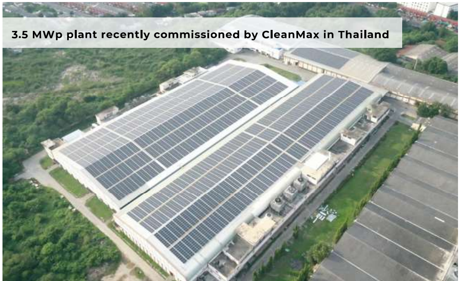
3.5 MWp plant recently commissioned by CleanMax in Thailand
